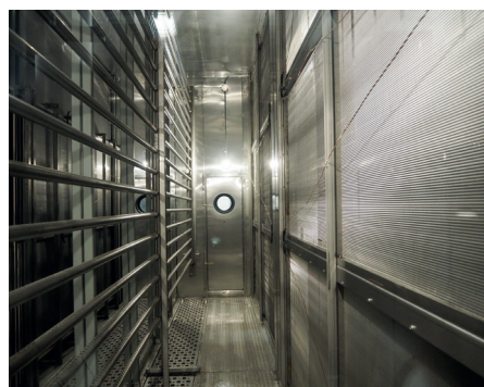
Internal view of the ventilation unit. On the right of the picture you can see one Konvekta heat exchanger.
