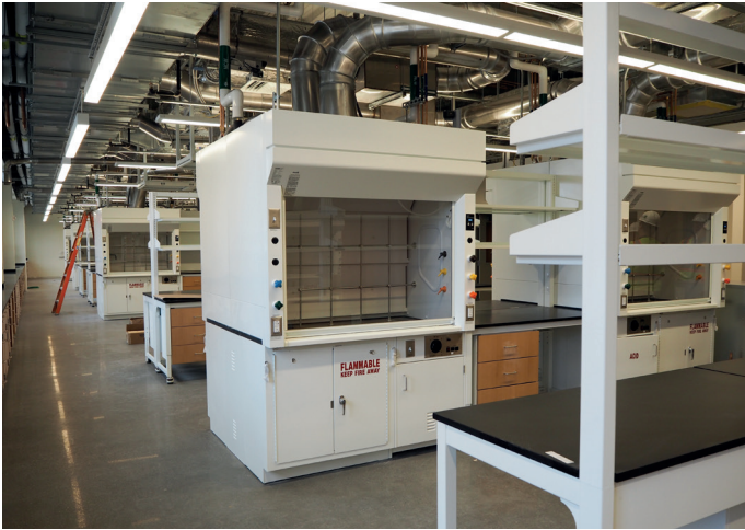
Digesters in the research laboratories for chemical tests. The exhaust air is drawn upwards and directly integrated into the exhaust channel. This means the contaminated or dangerous exhaust air is immediately exhausted.
