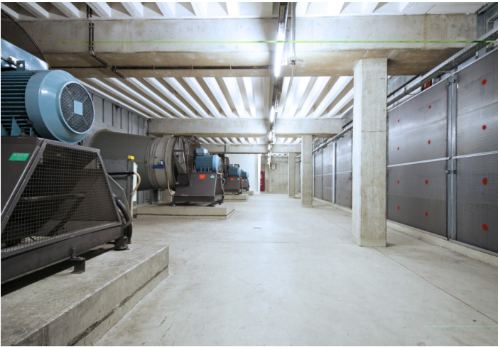
Supply air station for 470,000 cfm: four existing ventilators with blade adjustment supply the building with the necessary outside air.
