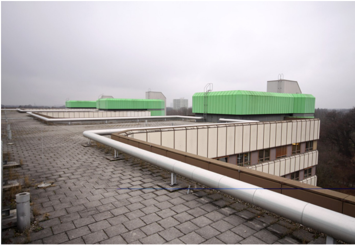
The piping system (according to Tichelmann) from 1979 combines ten exhaust air stations on the roof with the supply air station on the 2 nd basement floor.
