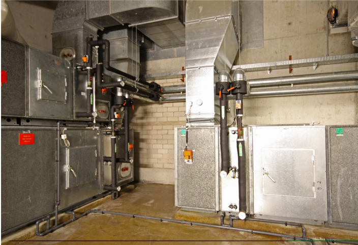
The heat recovery air coolers, connecting ducts, controls and stop valves were completely replaced in the course of the RAERS upgrade.
