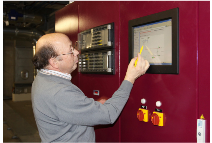
All data from the heat recovery controller can be accessed on a touch screen. Photo: Albert Holzbauer, longtime heat recovery system attendant.
