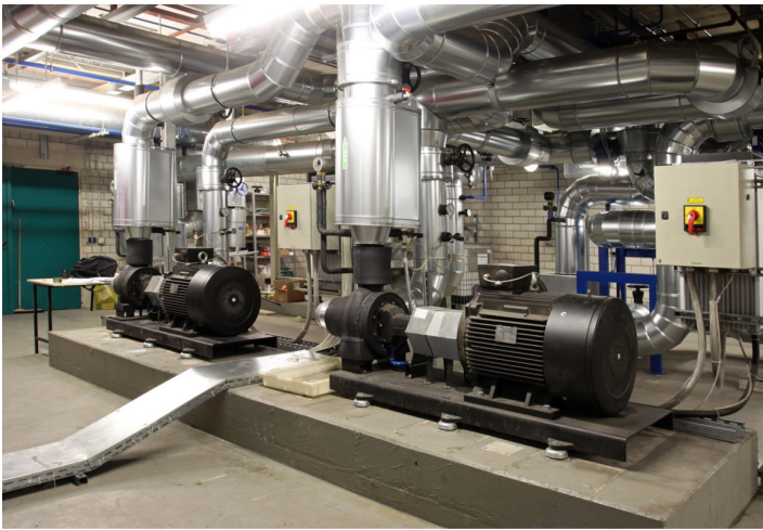
Instead of eight pumps, today two circulation pumps controlled by frequency converters provide an energy and performance optimized flow.
